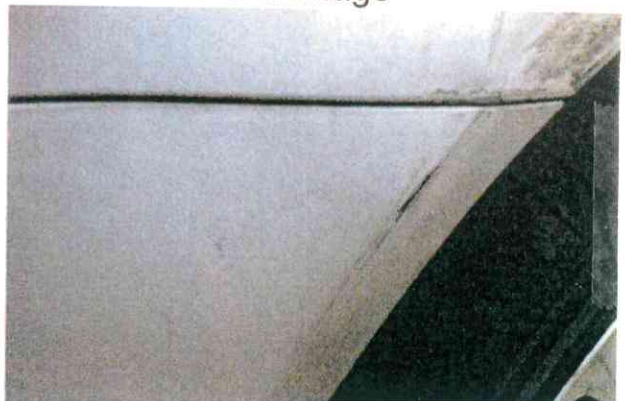
Closer view of damage
